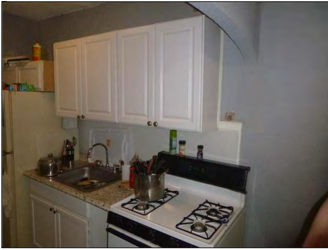
4.4 1 Loose wall cabinetry in 302
