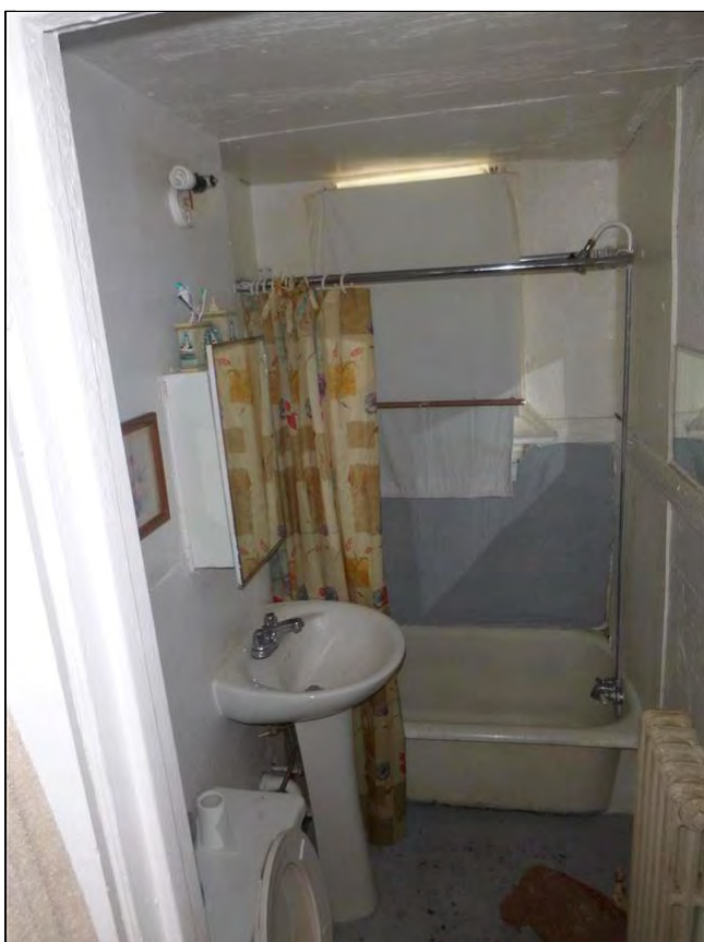
7.1 3 101 - Paint is not adequate to prevent water penetration
