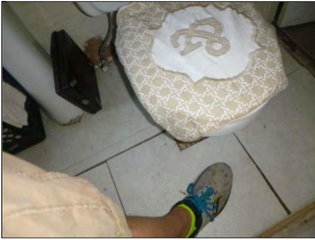
7.1 6 305 - the floor is pretty sketchy under this one (5) Loose bathroom sinks in 202, 204, 302. Secure to wall properly as needed
