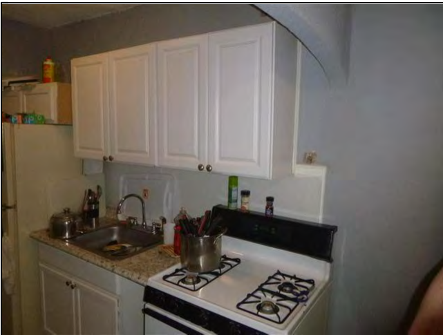
4.4 1 Loose wall cabinetry in 302
